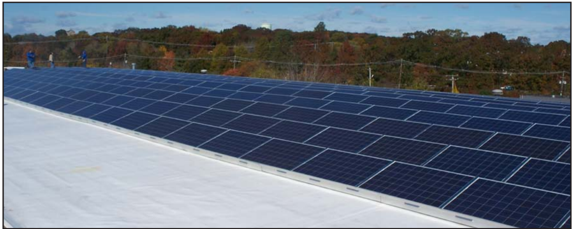
The system consists of 299 solar modules panels along with an innovative ballast mounting system which does not penetrate the roof.
